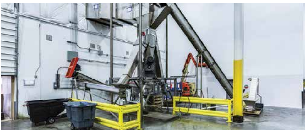
Integrated waste and recycling center with zero landfill target
